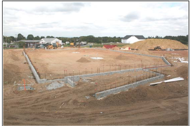
The CVS/pharmacy currently under construction, is scheduled to be completed in early 2010.
